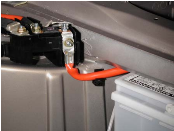
Junction point with 120mm 2 aluminum flat cable , 250 Amp fusible link (F-200)
